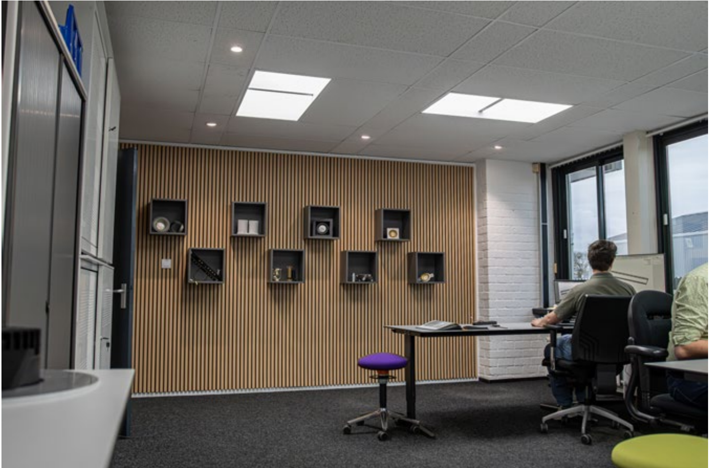
The lighting plan consists of two lighting groups. The panels provide a high mDER value for the eyes, while the downlights create comfort for the employee. Both groups operate independently to create a dynamic atmosphere.
